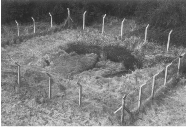
Figure 2.29 Collapsed mine shaft at Carrickfergus, Northern Ireland.
